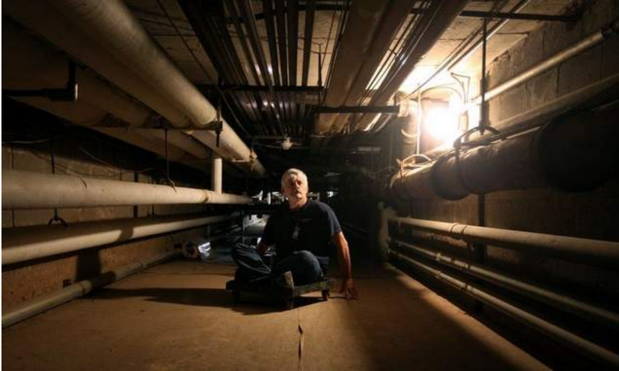
Scott Wilson, head building custodian, rolls through a small space in the walls of Barclay Elementary School in Brockport. Most of the piping in the school is still wrapped in asbestos. / JAMIE GERMANO / staff photographer
